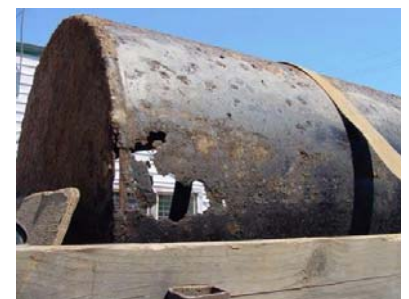
50 year old rusted heating oil tank
